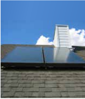
Vitosol 200-F flat plate solar collectors
